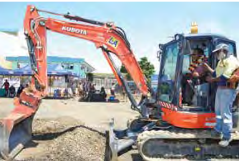
Governor Bakani CMG 'hands-on', participated in the ground-breaking ceremony of the Lae Currency Distribution Facility.
